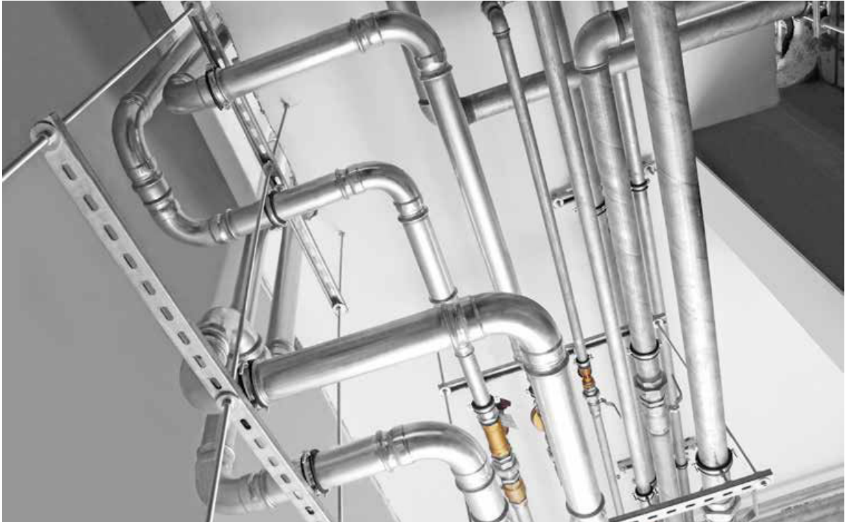
Exemplary KAN-therm Inox installation
