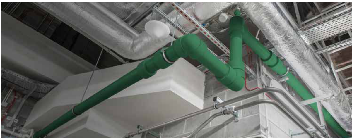
KAN-therm PP Green installations
