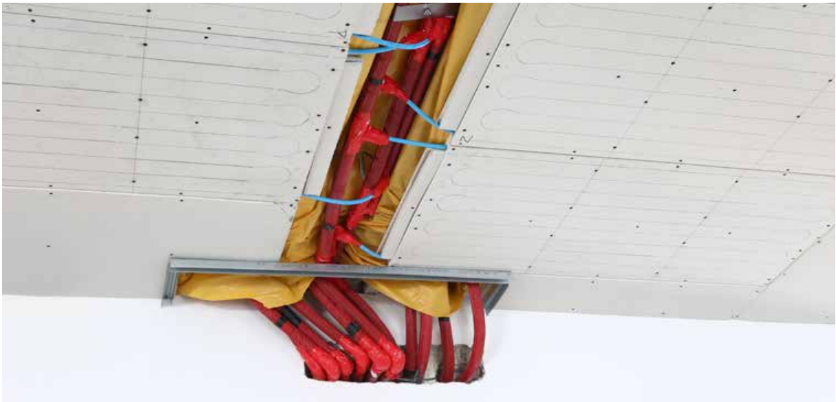
Fig. 6. Ceiling cooling installation using heating and cooling panels of KAN-therm Wall system.
