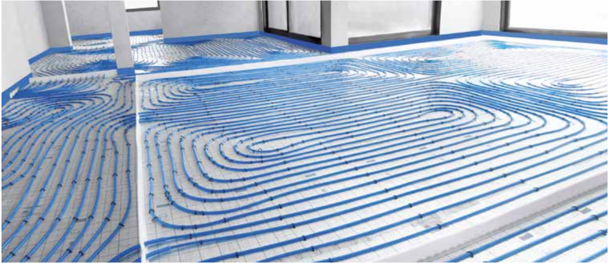
Fig. 25. KAN-therm Tacker system floor heating/cooling.
