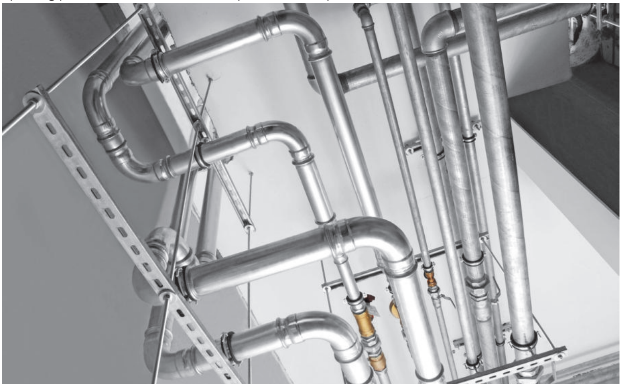
Exemplary KAN-therm Inox 304 installation
