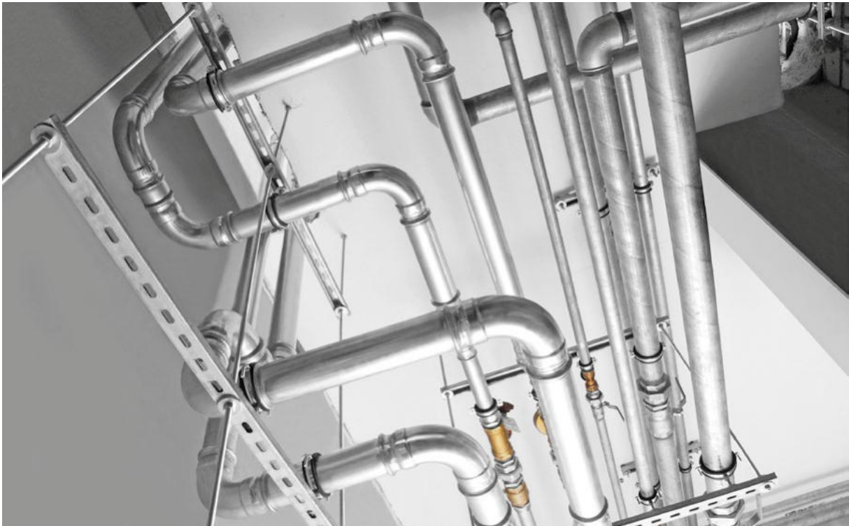
Exemplary KAN-therm Inox installation
